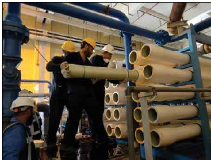
Picture 5. VONTRON membranes being loaded
