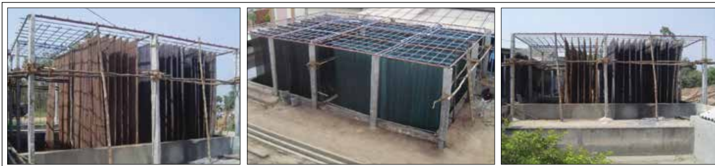
Fig. 2. The Net Evaporator System at M/S Suntex Processing Mills, Chennai. The nettings, basin and feed grid pipe on the top is fed by submersible pump inside the basin.
