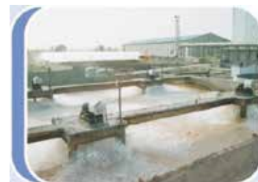
Effluent Treatment Plant
