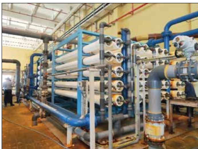
Picture 3. Sea water RO system
