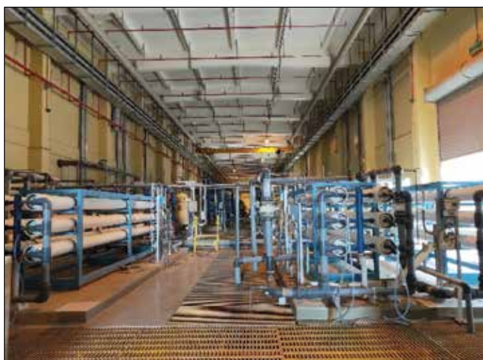
Picture 4. 2nd Pass RO system
