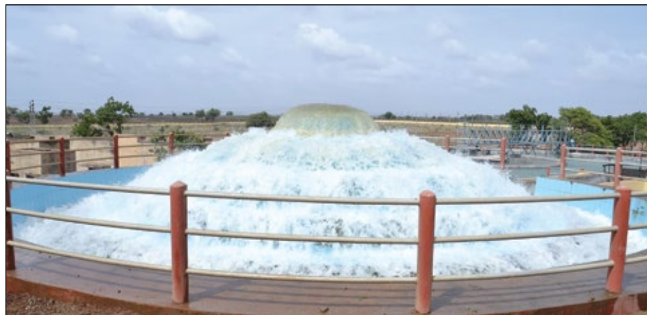
68 MLD Water Treatment Plant, Hubli-Dharwad, Karnataka
