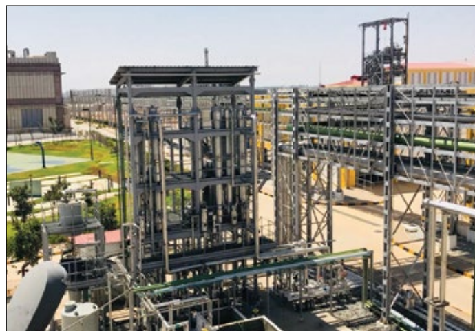
Zero Liquid Discharge plant installed by Thermax
