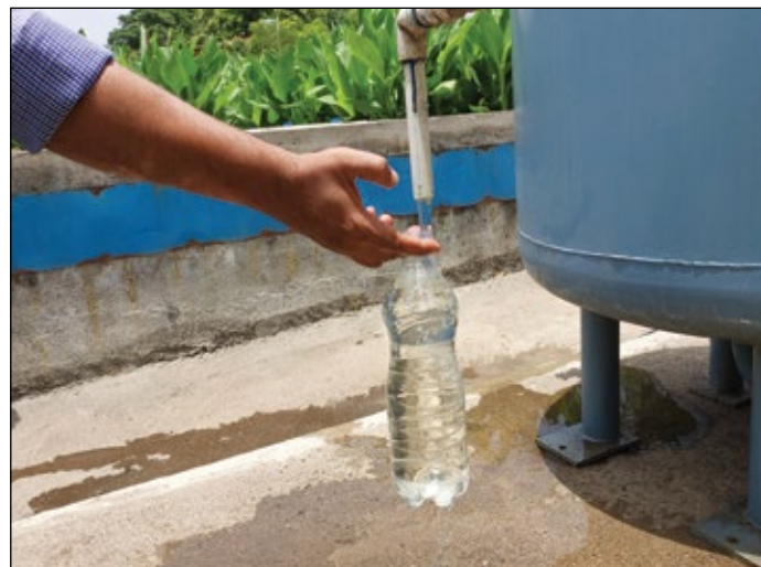
Final Treated water from the ETP
