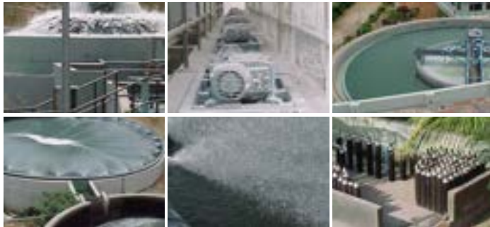
Fig.6 Modified WTP - Clockwise from top left, Cascade aeration, Lime dosing, High lime water clariflocculator with rapid sand filter in the background, CO 2 cylinders, NH 3 stripping sprays and the same tank in far ground dosed with CO 2 at the floor level by tubular diffusers.
