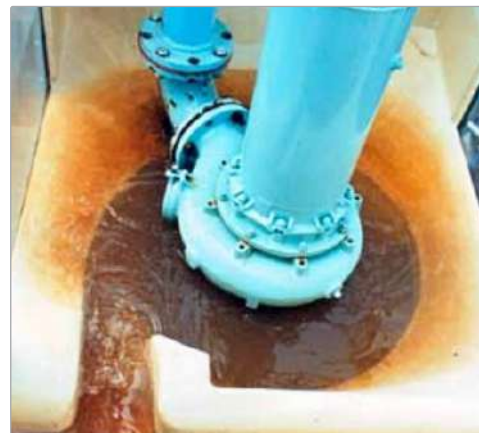
Fig.3. The Immersible Pump showing volute flow to the suction and the dry floor (3)
