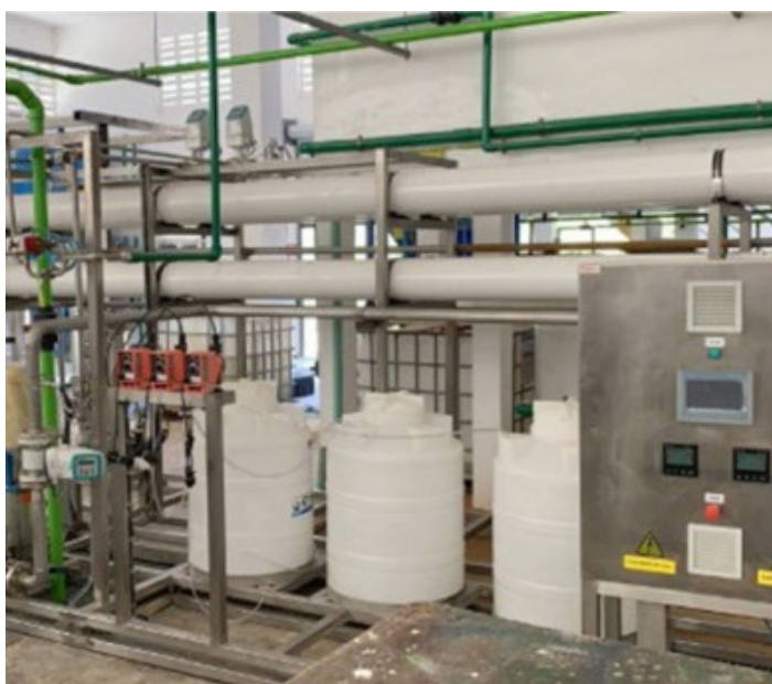
Nano filtration system
