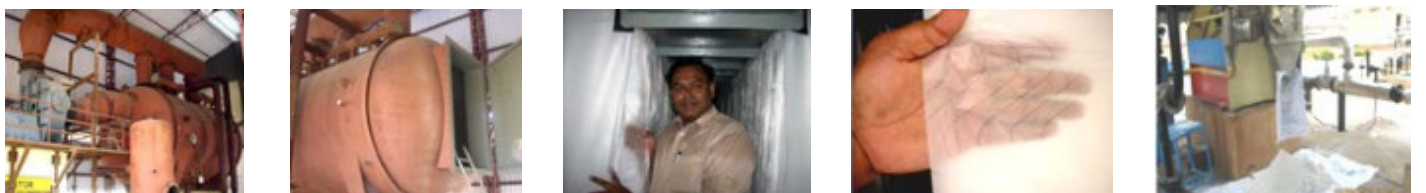
Fig. 3. The Mechanical Vapour Compressor Evaporator. The calendria spalling issues are overcome by synthetic sheets demonstrated by the second author and the typical final centrifuge to get at the salt
