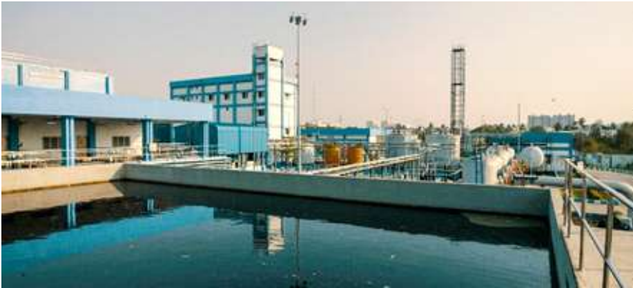
Koyambedu wastewater treatment plant in Chennai, 22% reduction in energy consumption with use of Danfoss VFD's for pumps, mixers, blowers, and dewatering applications.
