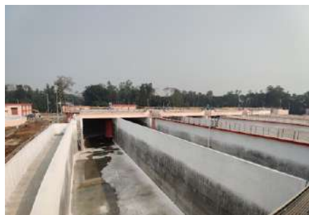
Fig.2–Ovivo's advanced Oxidation Ditch Site Image
