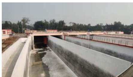
Fig.2 Ovivo's Advanced Oxidation Ditch Site Image
