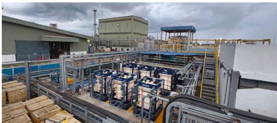
INDRA's wastewater treatment plant | Source: INDRA
