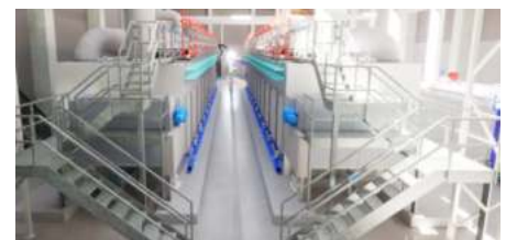
2 nos. HUBER Belt Dryer BT 22 in Roeselare. (© HUBER SE)
