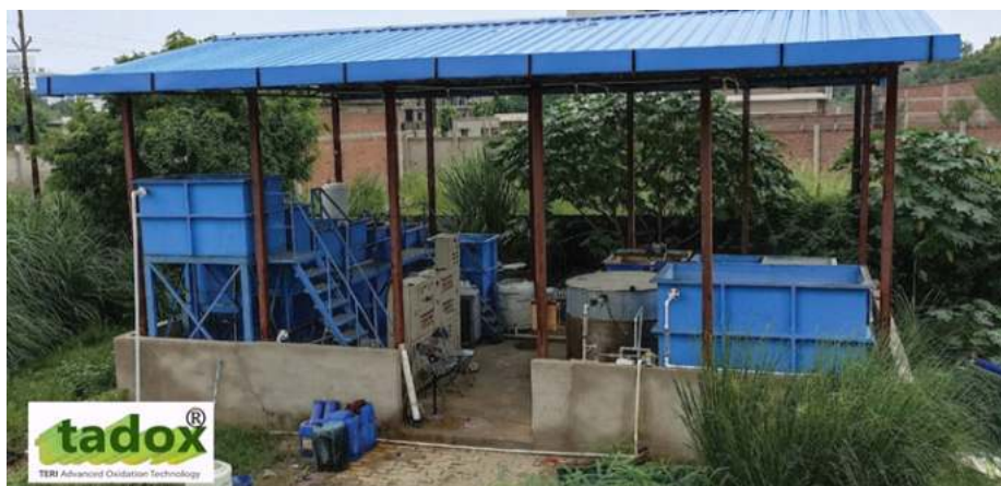
Figure 2: 20 KLD TADOX® Plant in the textile CETP.
