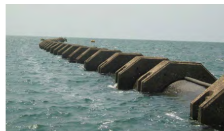
Photo 1. PE Pipe 1600 mm, Seawater intake pipe at Chennai, Desalination plant.
